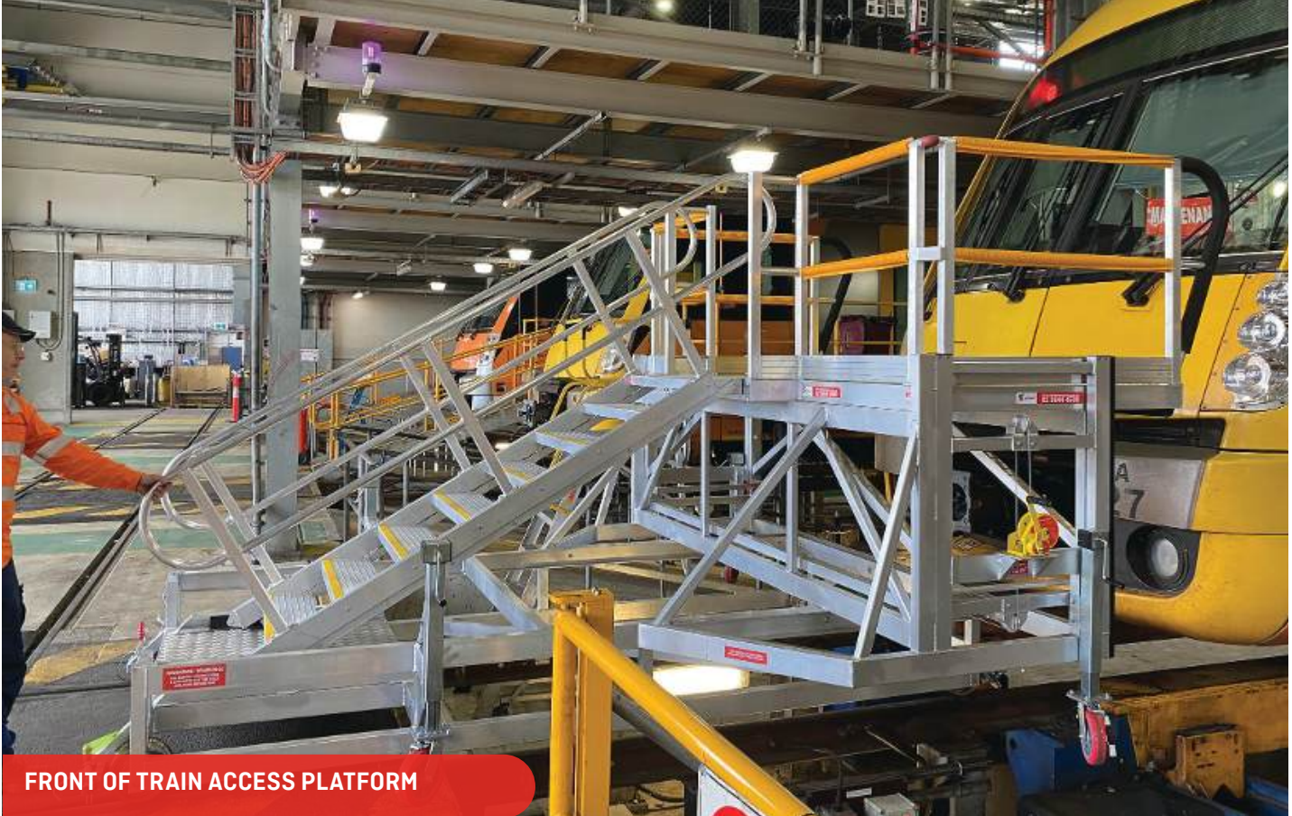
FIXED COUPLER ACCESS PLATFORM
